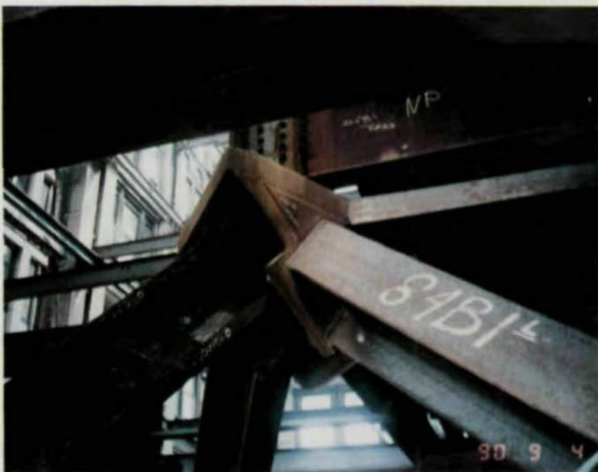
The joints in the transfer system were designed to direct the load into the diagonal and thereby control overload to the nearest column.
