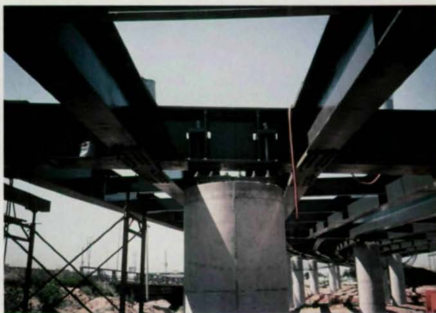
A continuous welded plate girder system was chosen as being the most desirable in terms of cost and aesthetics, as well as having very low maintenance requirements.
