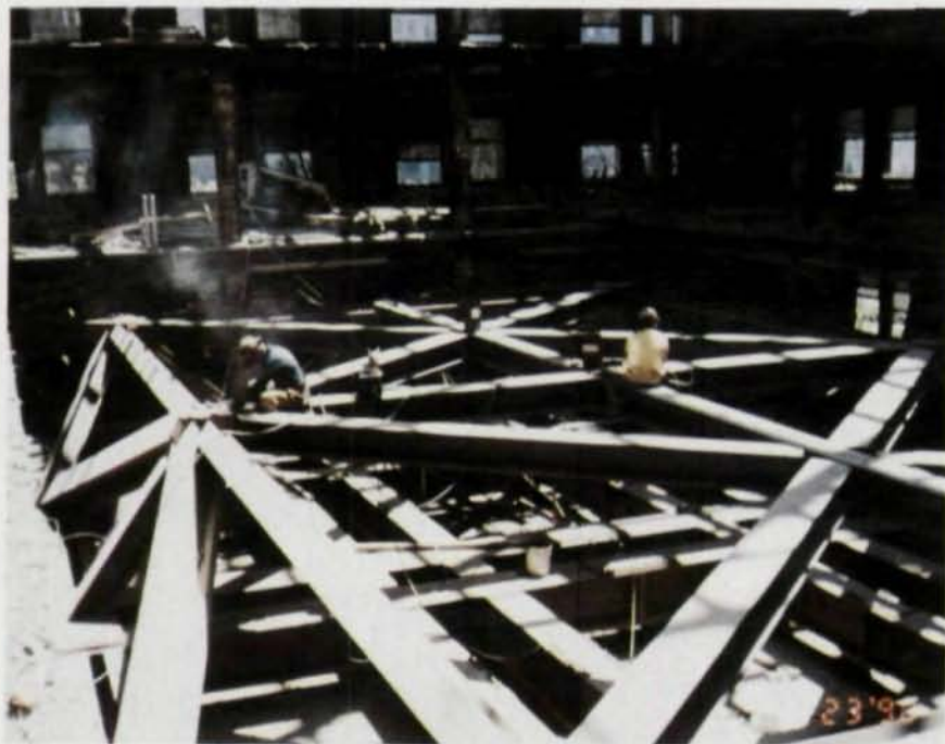
The superstructure supports the six new core columns and transfers their reactions to the lower grid.
