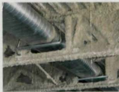
The Vierendeel opening in the joist allows easy placement and routing of major mechanical ductwork.
