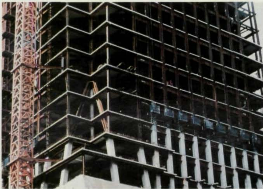
A unique sloped column system occurs between the 10th and 13th floors of Mellon Bank Center, where the four inside corner columns are picked up on a "two-legged tripod." Each "two-legged tripod" generates significant lateral forces that are all balanced out by balancing one corner against the opposite end.
