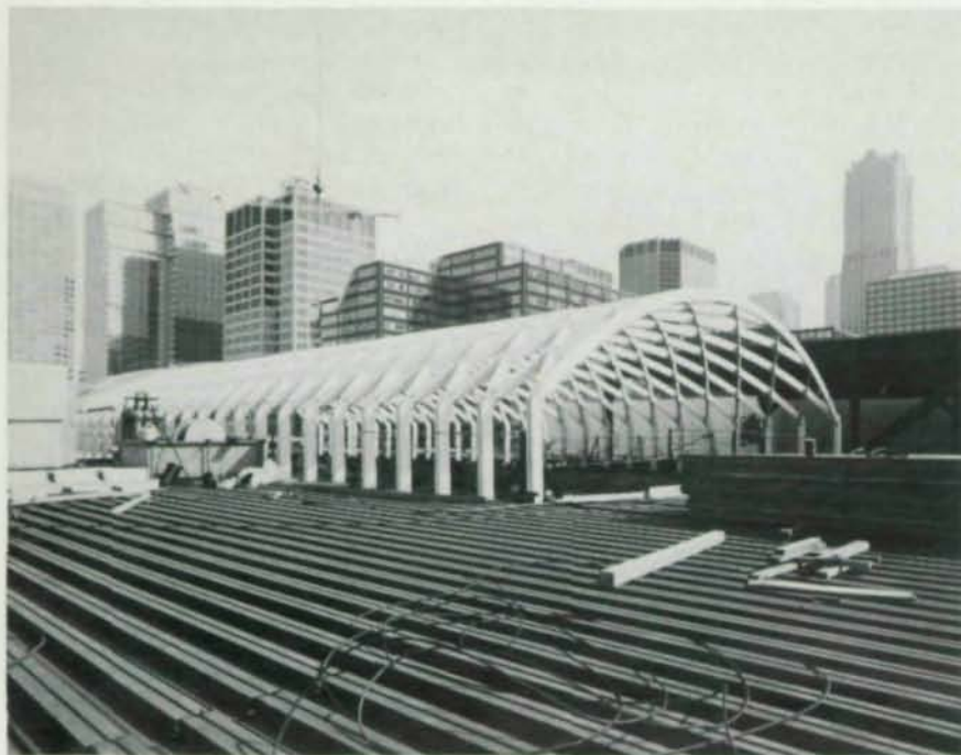
The space frame consists of 10" x 2" x 1/4" tubes with nodes made of 3"-diameter extra-strong pipe. The frame has a radius of 36" and lateral thrust on the roof structure is taken by adjacent framing members. Photo by Mc Shane Fleming Studios.
