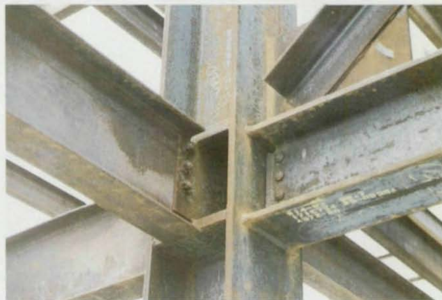
Seismic resistance is becoming increasingly important for hospital projects throughout the United States. Shown at top is a partially erected frame for a new hospital in California. The connection shown above is for a project in a high seismic area.
