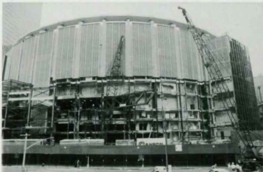
In order to create a full-size stage for the Paramount Theater, an addition was added on the Eighth Ave. side (top). Because the creation of the new stage required the removal of two columns, large trusses were required to pick up the building load. However, the only available location for these trusses was between the fifth and sixth floors (above).
