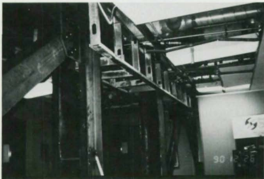
Shown at top are workmen bringing steel into the existing building through a ninth floor window. Bottom photo shows the bulkhead framing. Photos courtesy of Eli Lilly.
