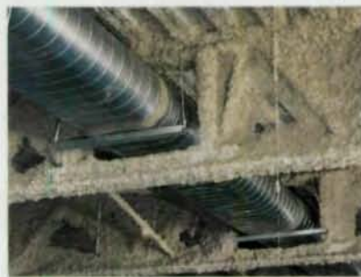
The Vierendeel opening in the joist allows easy placement and routing of major mechanical ductwork.
