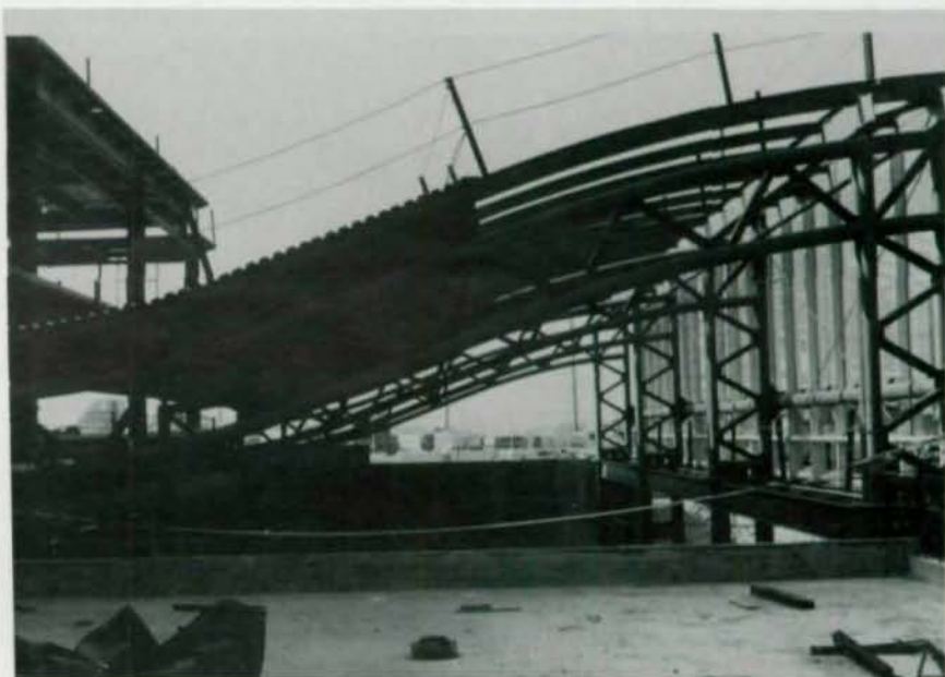
AWS D1.1 provides detailed information on welding and inspecting "T" and "K" joint pipe-to-pipe connections that allows the clean welded connection of structural pipes without cumbersome gusset plates or back-up bars. As shown above, the web angles are welded to semi-circular vertical plates that transfer the axial tension and compression forces back to the pipes via three horizontal plates. Shown on the opposite page are curved pipe elements forming a partial arch in the F.I.S. section of the structure.
