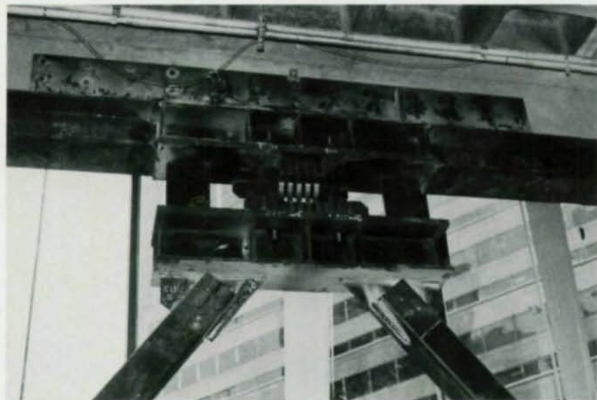
The photos above show an Added Damping and Stiffness (ADAS) element during fabrication and after installation in the Wells Fargo Building in San Francisco. The unit includes five 1.5"-thick 50 ksi steel plates clamped together with A490 bolts.
