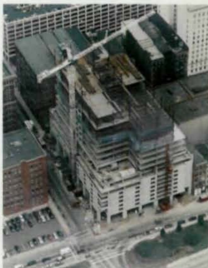
An added benefit of the selected framing system was the rapid, 56-day erection period.
