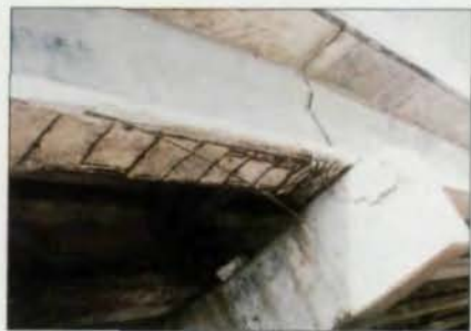
Durability of concrete is an increasingly serious issue. The decline of the load carrying capacity of deteriorating concrete road bridges is not yet fully understood.
