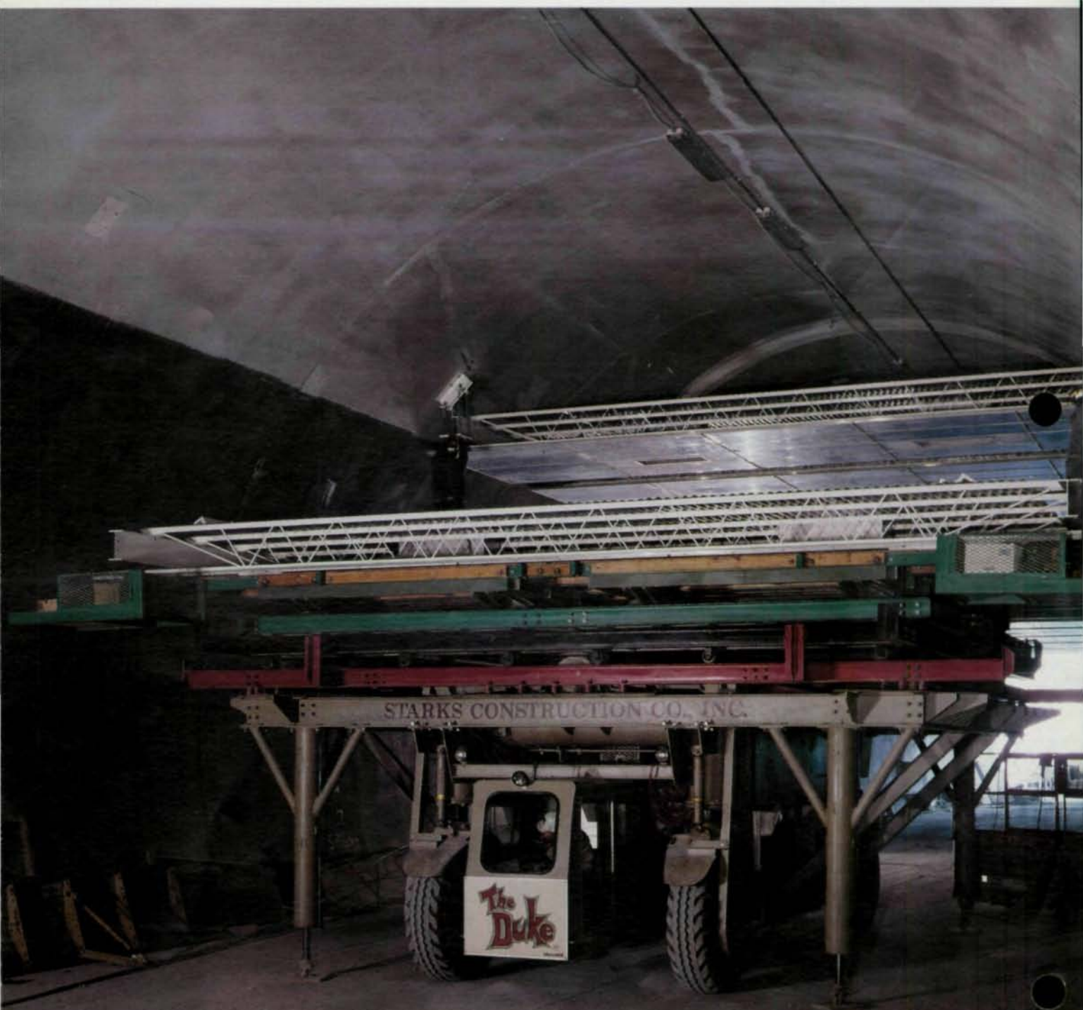
The "Duke" installing ceiling panels in the Hanging Lakes Tunnel, Glenwood Canyon, Colorado.
