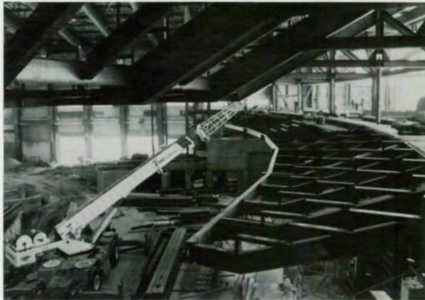
The cantilevered balconies were supported on a pair of new steel columns. Photo by Kent Bolerjack.
