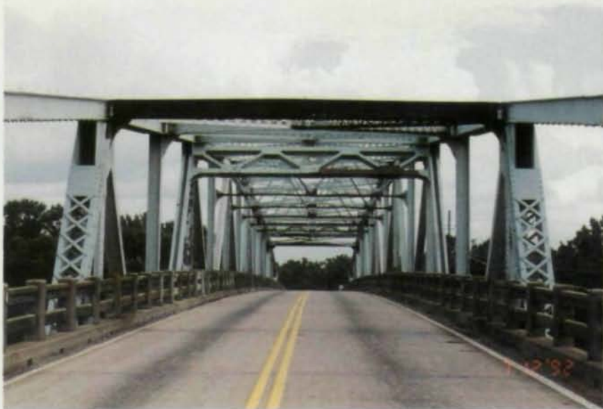
Pictured above is an end view of the bridge channel span of the Apalachicola River Bridge. Under the proposed retrofit scheme, some of the sway bracing would be replaced in order to increase the overhead clearance.
