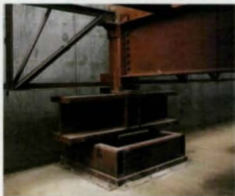
The design team chose a "base isolation" system to accommodate seismic loads. They also specified Vulcraft steel joists and joist girders for the building.
