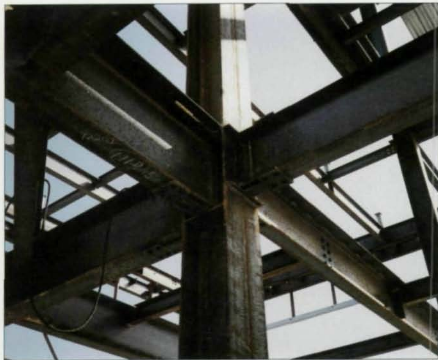
Semi-rigid beam-to-column connections, such as those shown above and opposite, were used on the new two-story hospital addition at the Deborah Heart and Lung Center.
