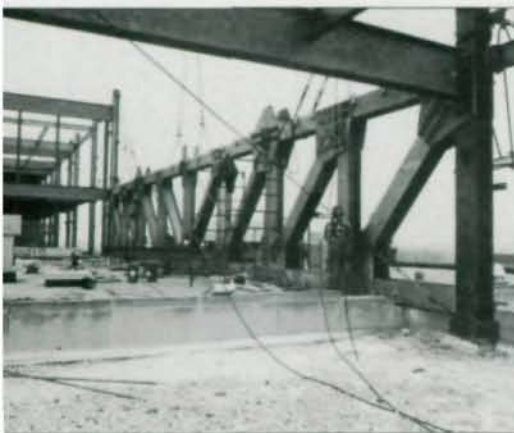
The hospital's vertical addition was constructed with wide-flange members instead of trusses largely to simplify fireproofing.
