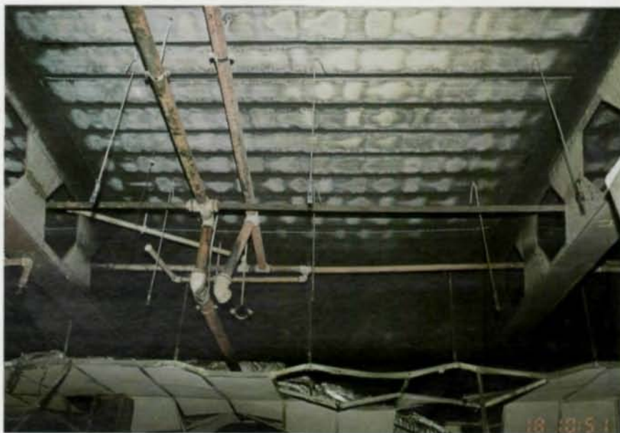
Shown at top is the test structure prior to the fire. The photo above shows the results of the fire: While the ceiling system was destroyed, the steel structural system was largely unaffected.
