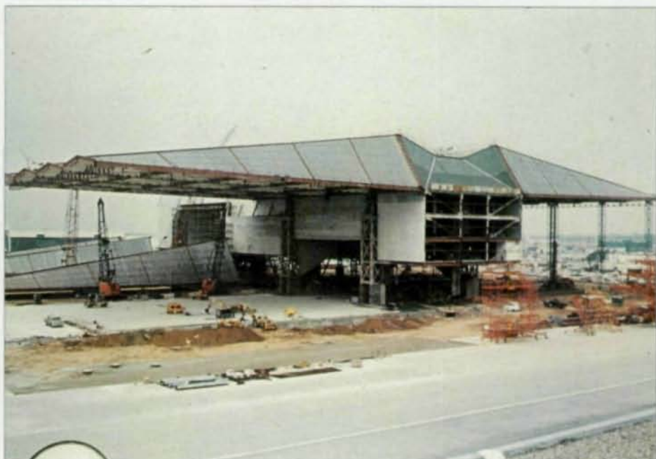
Zetlin's student and colleague, Charles Thornton, considers the American Airlines Hangars in San Fransisco and Los Angeles to be his teacher's most innovative structures. The hangars have modular roof sections with cantilevers that extend 230' (70mm) from the core structure. The parabolic shape of the roof allowed room for airplanes to be raised off the ground during maintenance work.
