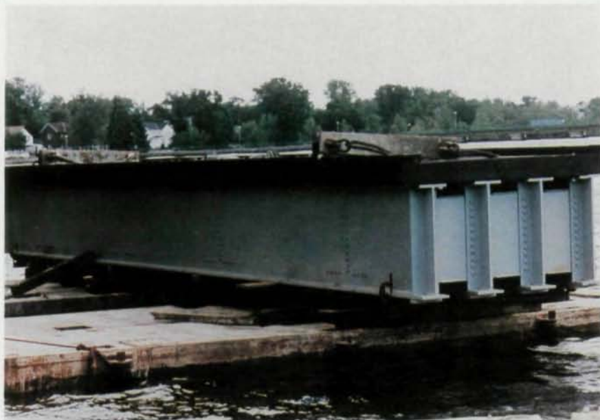
New spans for the Green Bay & Western Railroad Bridge were fully assembled on shore and loaded onto barges for final transport to the bridge site.
