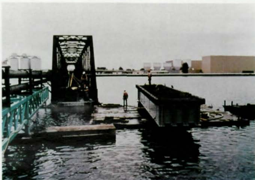
Each fully assembled span was floated into position and lowered onto the bearings by pumping water into the barges.
