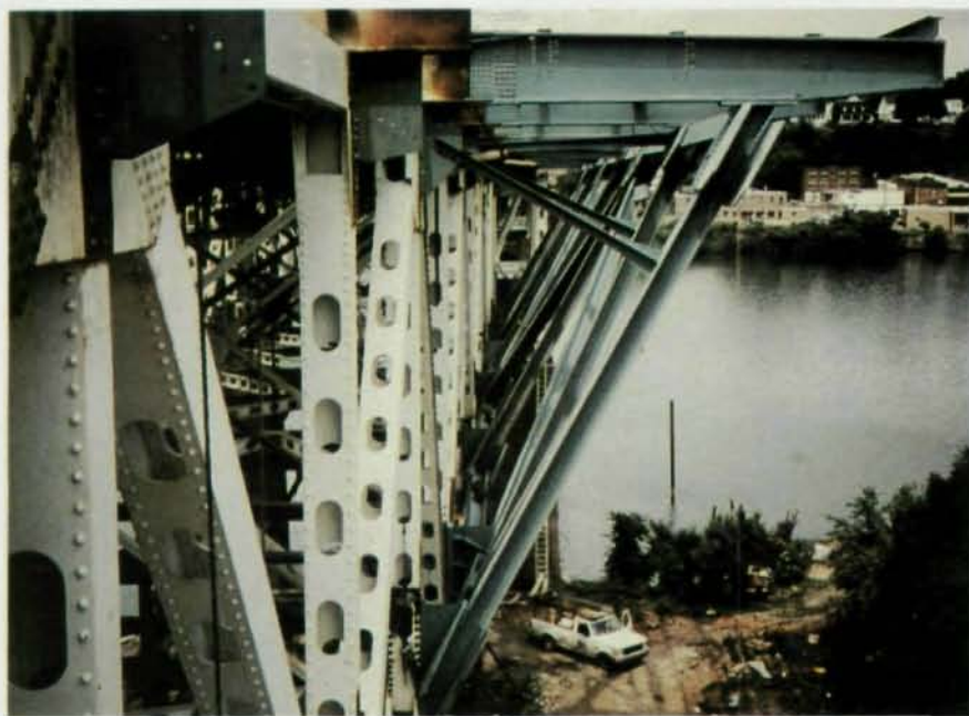
Pictured above are the new floor beam extensions supported on the sloped truss.
