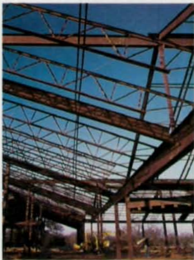
Sloped seat joists work in even the most complex customized framing jobs.
