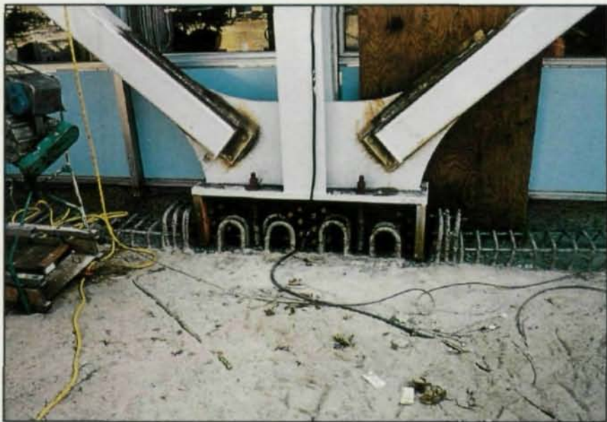
An external steel frame was used to bring this laboratory building up to current seismic code level.
