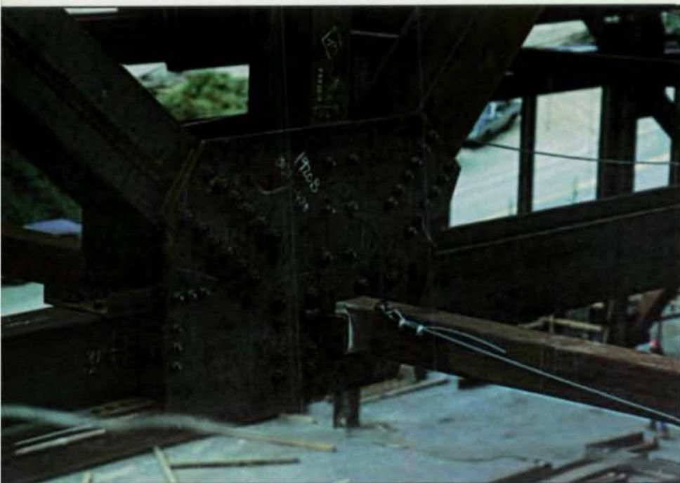
Shown is a closeup view of the first bottom chord connection out from truss to column top chord connection. Photo by Steven G. Hall
