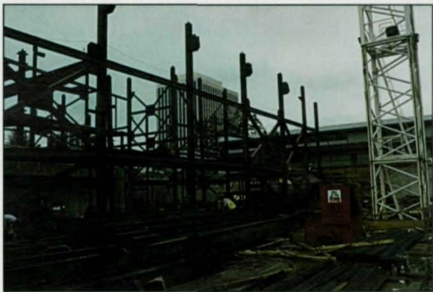
Shown on top is the main atrium between the theater and the exhibit hall. Pictured above is the braced frame. Note the large amount of steel girders on the exhibit hall floor slab. This is an example where construction loadings may be the highest a floor will receive. Photo, top left, by James F. Housel; photos, top right and above, by Steven G. Hall
