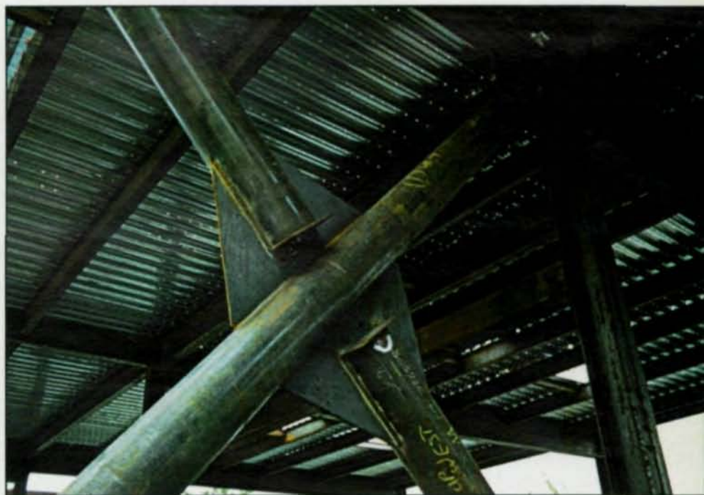
Shown is a closeup view of a braced frame. The brace members were typically slotted, held in place with erection bolts, and field welded to gusset plates. Photo by Steven G. Hall
