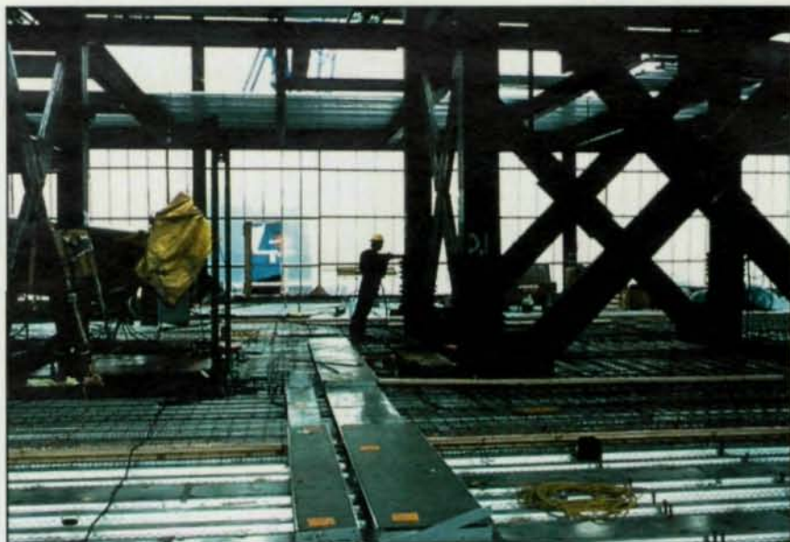
The Idaho Light & Power office complex in Boise features column-free floors. Instead, the columns are located external to the building shell. Structural steel X-bracing within the core walls resists lateral seismic and wind loads. Also, X-bracing was used around the elevator shafts instead of concrete shear walls.
