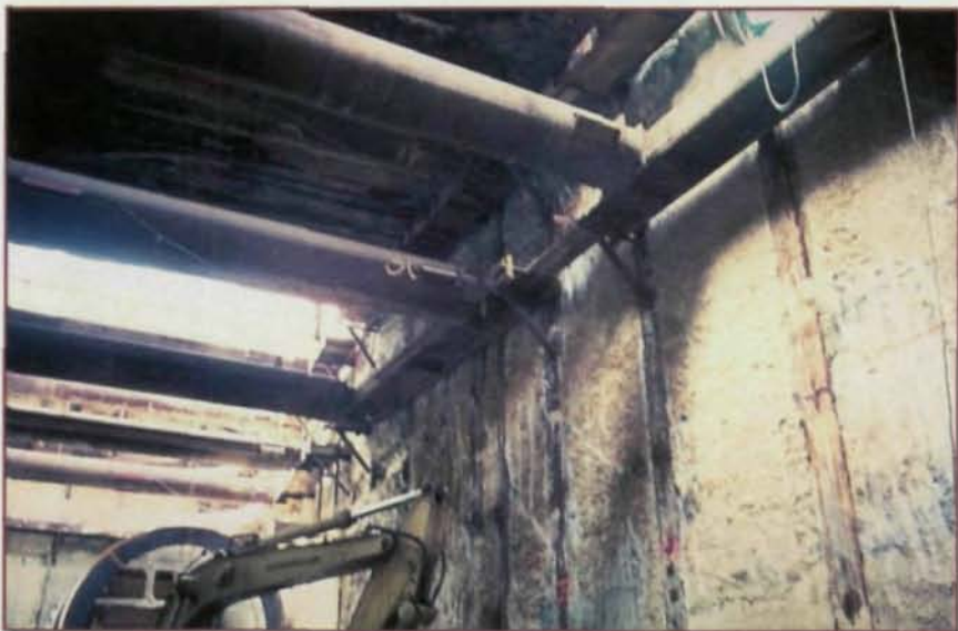
Pictured above is the construction of the Baltimore Shot Tower Station showing excavation, cross lot bracing and the SPTC wall. Pictured opposite is work on the Central Artery tunnel in Boston.
