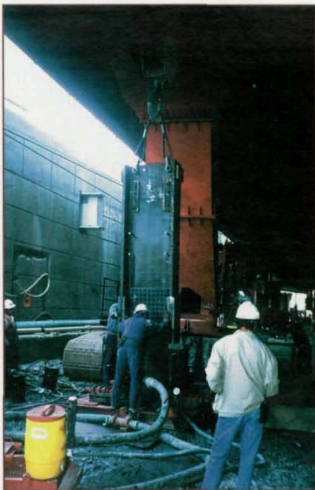
One of the difficulties with the Central Artery Project is the low head room beneath the existing Artery viaduct. Pictured is a soldier pile with bolted splices.
