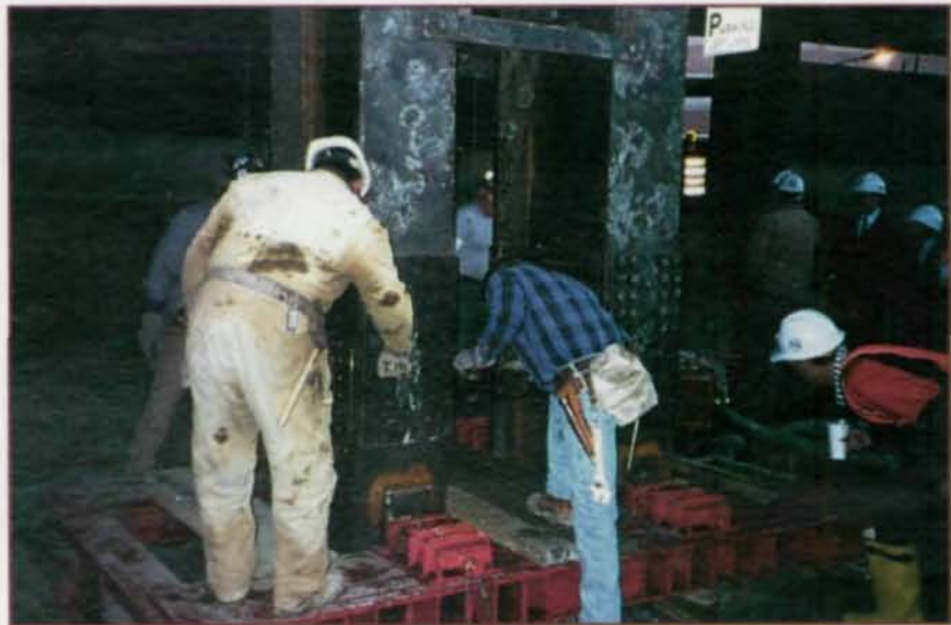
Because headroom clearance on the Central Artery tunnel project in Boston was only 20-ft., the 100-ft. long soldier piles needed a bolted splice detail utilizing A490 bolts.
