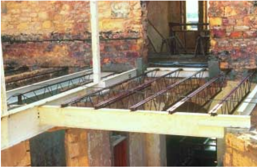
Shown above is the new second floor framing during construction. Pictured opposite is a view of some of the diagonal ridge and valley trusses, along with the stone chimney in the background.
