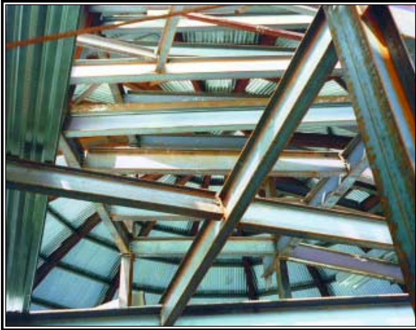
The photo above pictures five different levels of steel framing and demonstrates the complex and intricate design demanded in this project.
