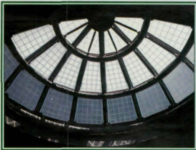
The Salt Palace—Salt Lake City's new Convention Center—utilized tubular members to frame its extensive skylight system.
