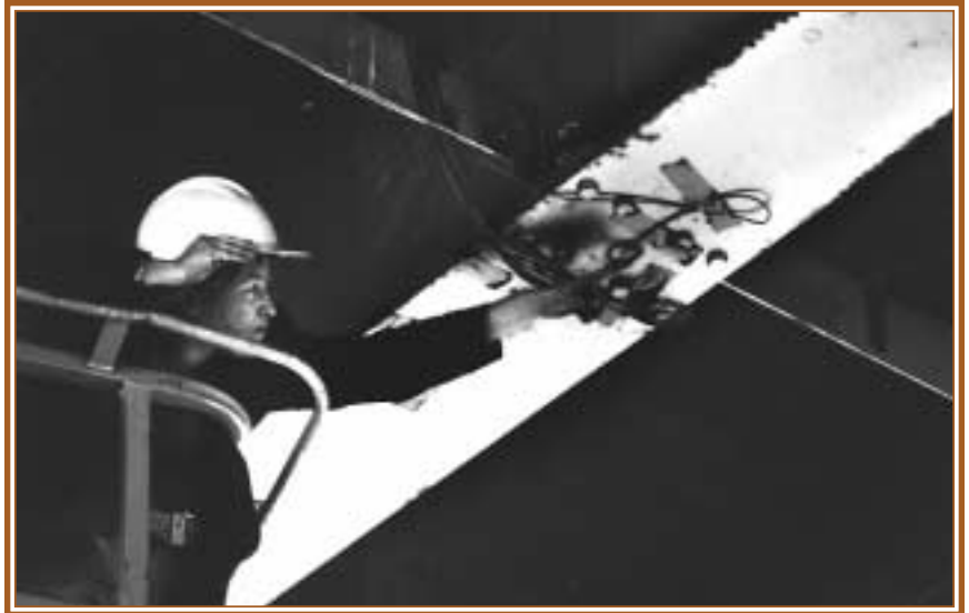
Rola Idriss, a professor at New Mexico State University, installed 30 sensors on a bridge in Las Cruces, NM, to test a remote-monitoring system.
