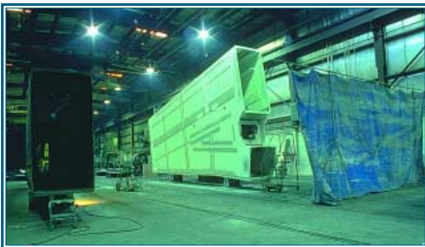
Shown above, from top to bottom: arch and cross-sections; elevation of "Y" joint; and shop assembly of "Y" joint.
