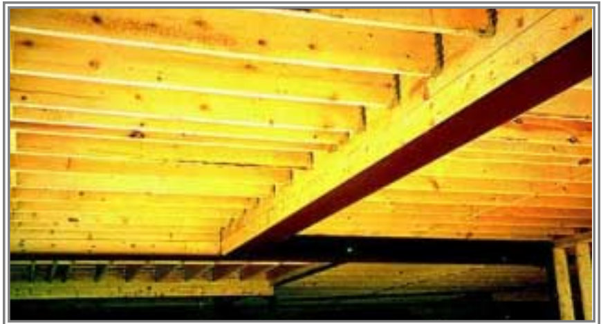
The Warren House in Woburn, MA, utilized steel to help create column-free space in the basement. Photos by Dimitri Papadimitriou.
