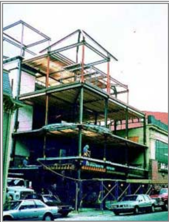
The Omni Travel Building also utilized both wood and steel for its structural system.
