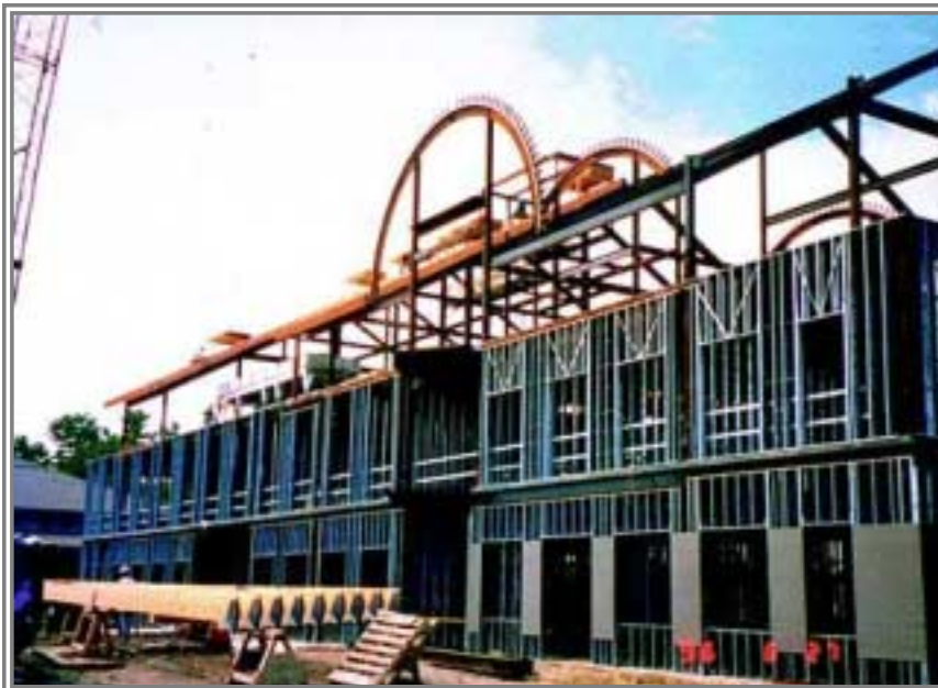
A combination of wood and steel proved most effective for the Geological Science Center at the University of Maine.
