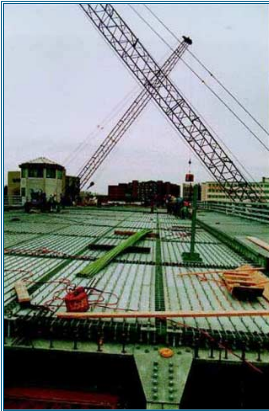
Another view of the Exodermic bridge deck system during installation on the Main Street Bascule Bridge in Green Bay,
