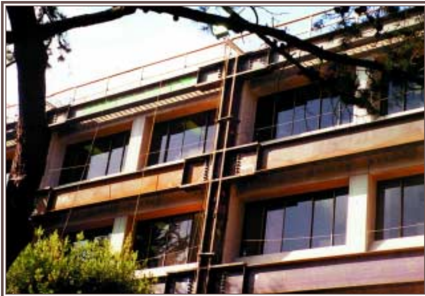
Pictured on top is a prefabricated column-connection assembly being lifted into position.
