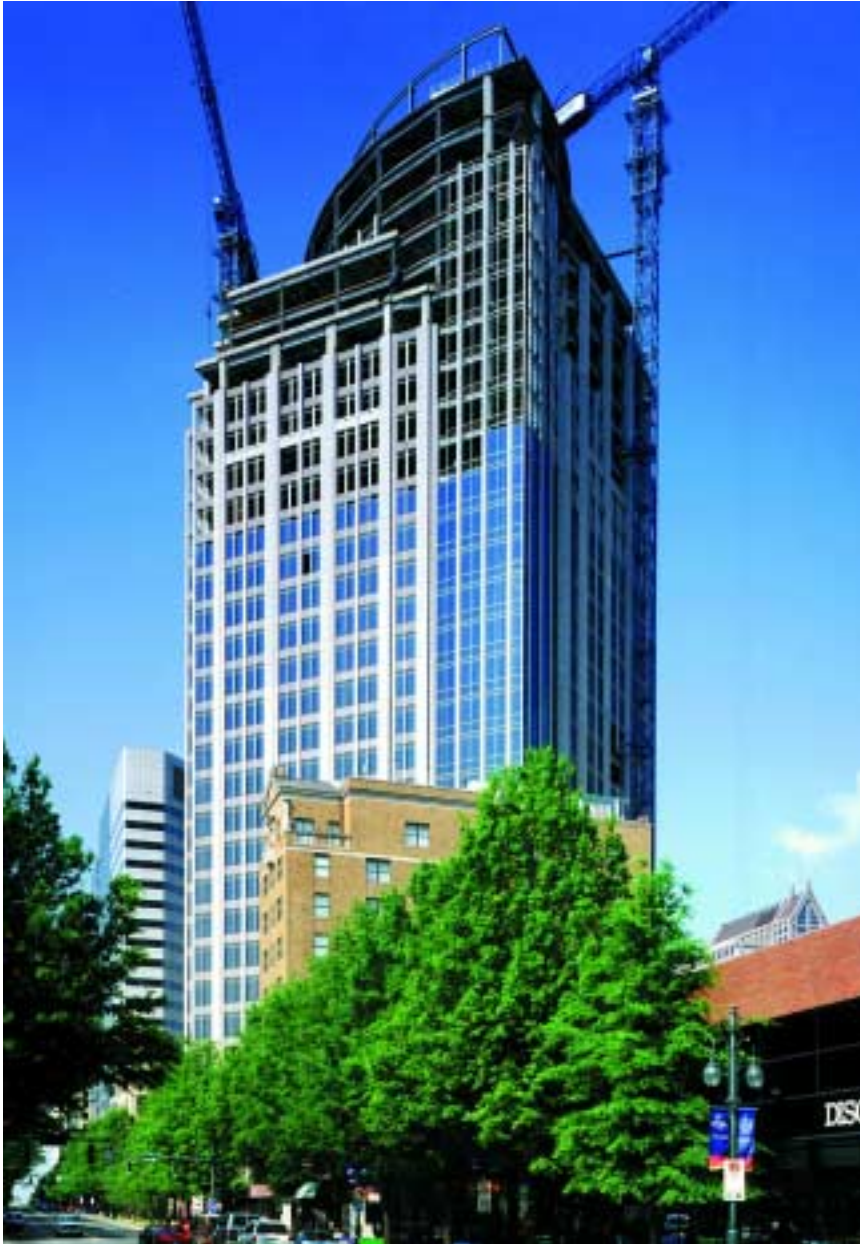
The 30-story IJL-Financial Center in Charlotte was designed with LRFD and utilizes concrete columns and steel girders.
