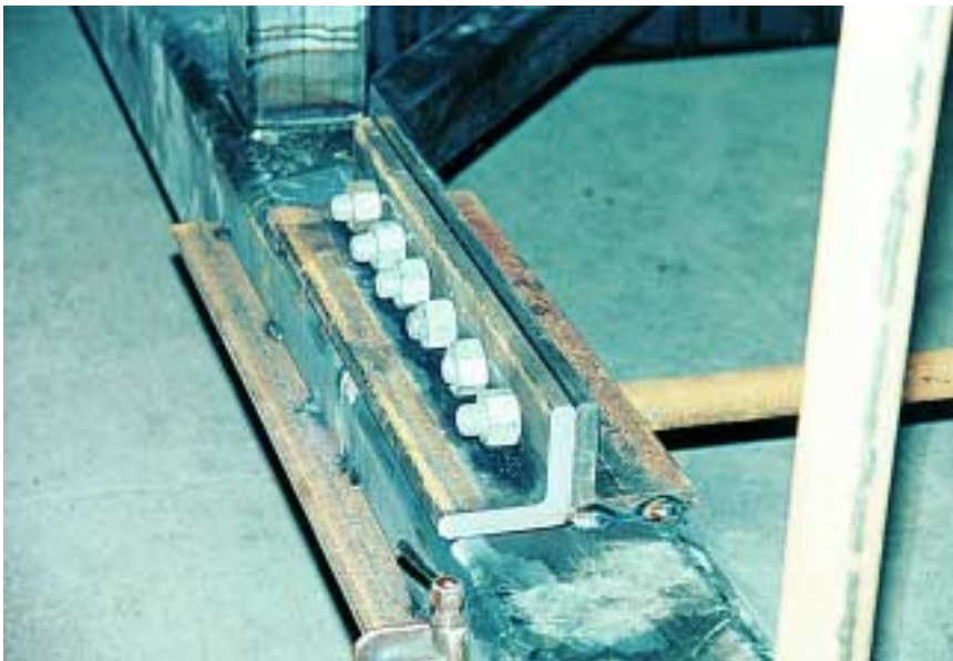
Trusses for the 82', 90' and 103' long spans were made in two sections, with a field splice in each of the four chords. After the tubing for the chord members were brought on-line, the splice locations were cleaned, bevelled and custom fitted with the backing material for the complete joint penetration welds (CJP) field welds. Alignment was achieved by using temporary "guide angles" for fit-up.
