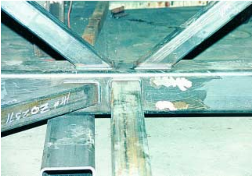
A high-level of craftsmanship was needed to meet the designer's aesthetic goals, which in turn required both careful fabrication and fit-up.
