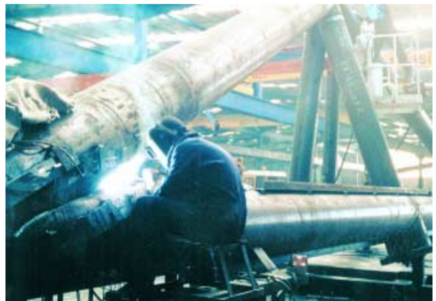
Top: After field welding, a tubular truss awaits installation as part of the retractable roof assembly.
