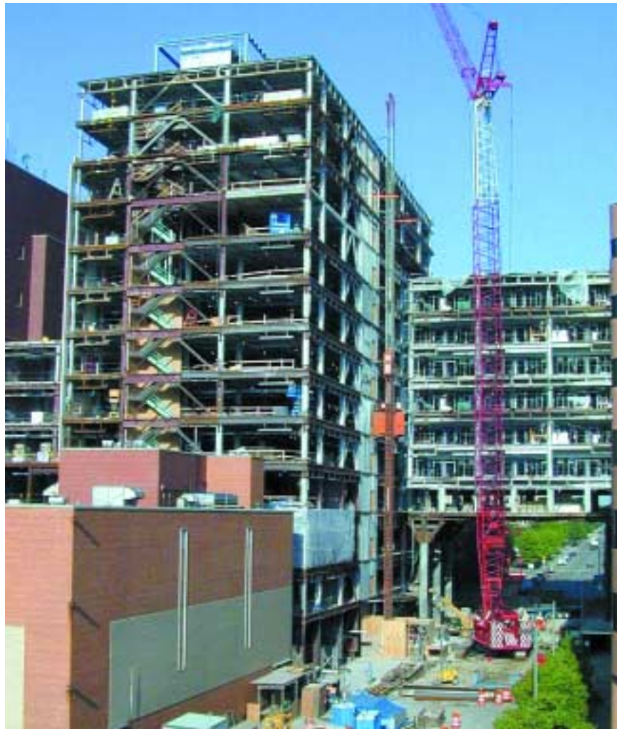
East elevation. Board of Water and Light building and Ottawa Bridge Building under construction.
