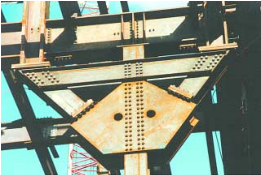
Closeup view of special v-shaped knee-bracing assembly to transfer forces from Vierendeel nodes to bridge support column.
