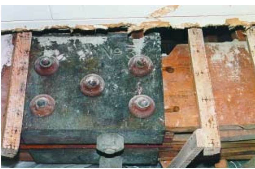
Dining room trusses had deflected substantially by 1938, prompting the addition of columns at the mid-span of each truss. This uncovered joint reveals significant structural damage.
