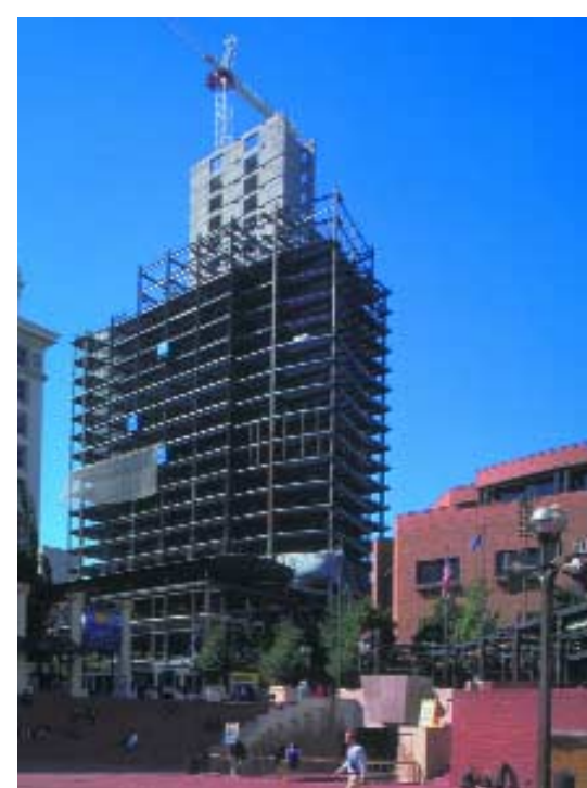
Construction of steel frame around concrete core elevator wall looking from Pioneer Square.
