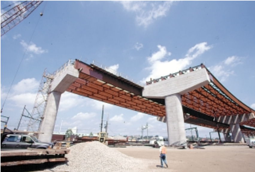
Steel girders on the Route 21 viaduct replacement are curved and must resist high torsional and seismic forces.
