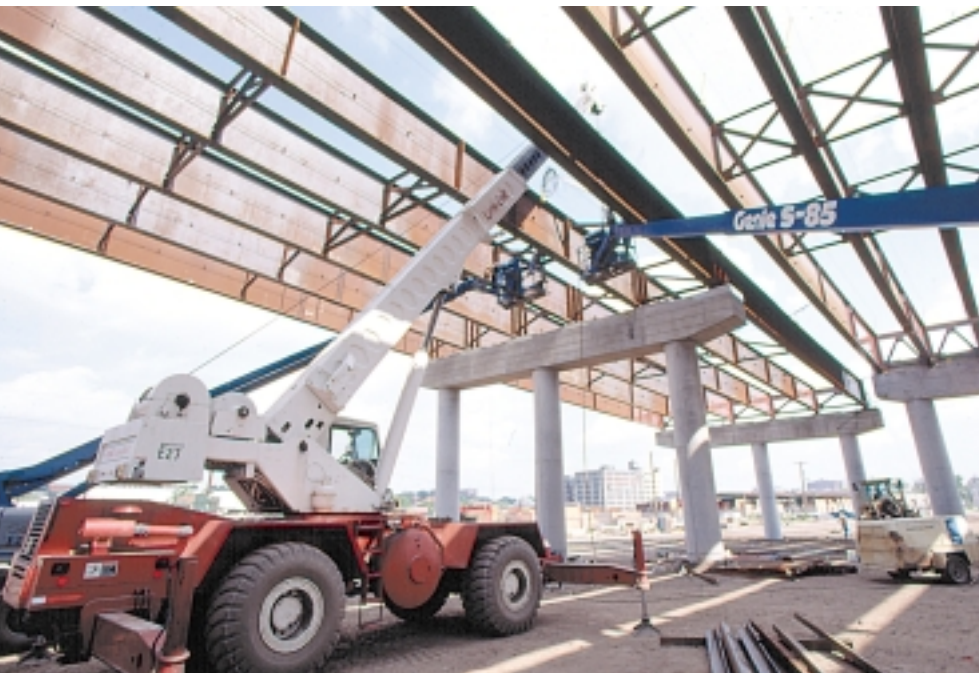
Cranes place girders for the southbound structure. The steel girders are 9' deep and reach spans up to 270' long.
