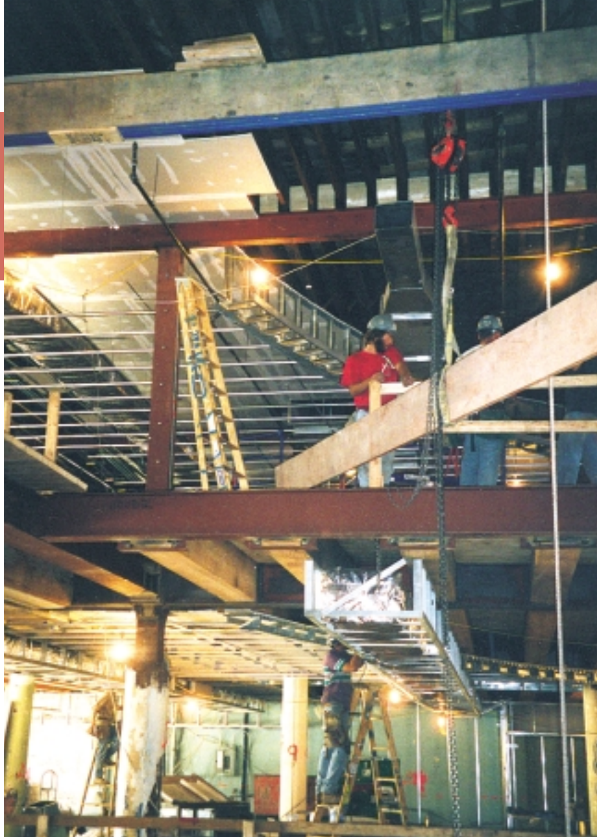
Steel members were used to create large openings in the existing bearing walls. Note the timber column, upper left, reinforced with channels bolted to both sides. Existing timber beams are supported with special seats welded to the steel girders.
