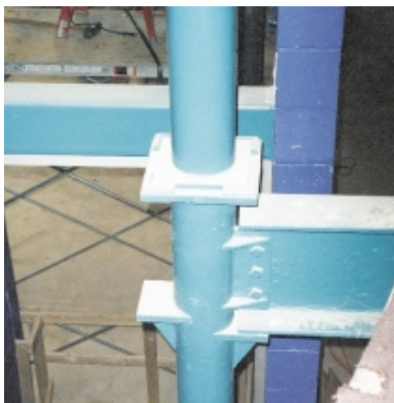
View of an existing cast-iron column-top connection. The existing columns have connection seats and web connection plates cast integrally with the column. The cast-iron cap plate has a cast "recess" to accept the column above.
