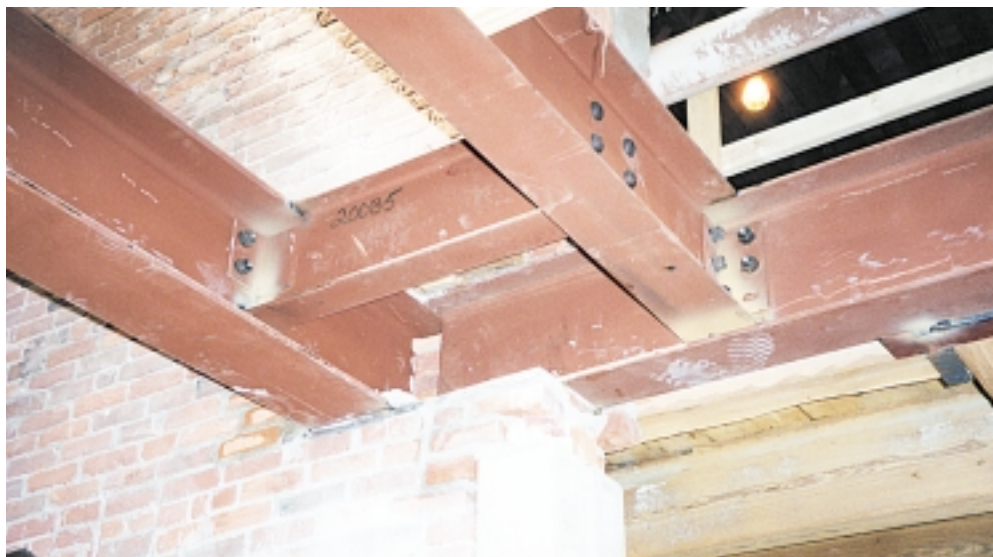
New escalator support beam (left). A "backup" beam, running parallel to the escalator support beam, helps resist torsion with a short, moment-connected filler beam.
