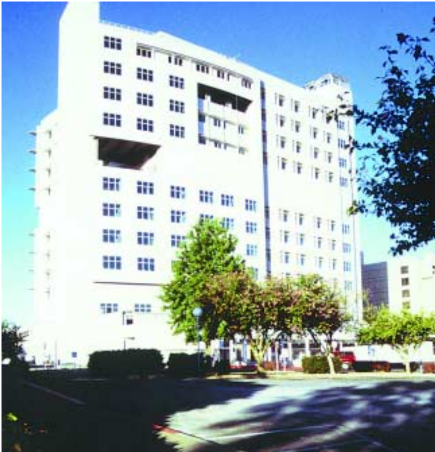
Top: Front elevation of the Davis Wing showing the more than 6,000 tons of structural steel near completion of erection
