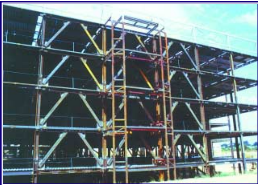
Steel frames and column bays of the VA Palo Alto Replacement Hospital
