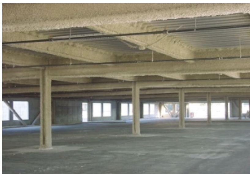
Interior of parking structure at Creekside Development, San Leandro, CA. The fire-protected beams and columns have not yet been finished with a troweled-on hardener.
