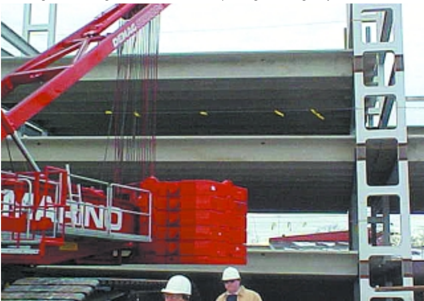
The Yale University School of Medicine parking structure under construction. Note the use of Hybrid Parking Solutions' prefabricated double-column sections to support precast concrete tees.
