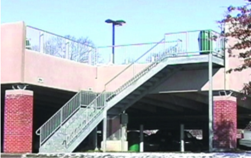
Access to the second level of parking at Bentley College is provided by galvanized steel staircases.
