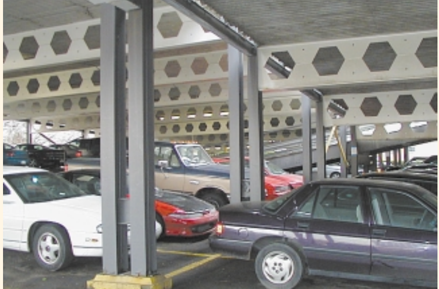
Recent photo of the 29-year-old Crickelwood Hill Apartments parking structure, Mulach's first steel-framed parking structure which still shows no signs of significant corrosion.
