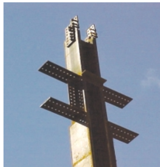
A typical column moment connection assembly for the lateral force resisting system.
