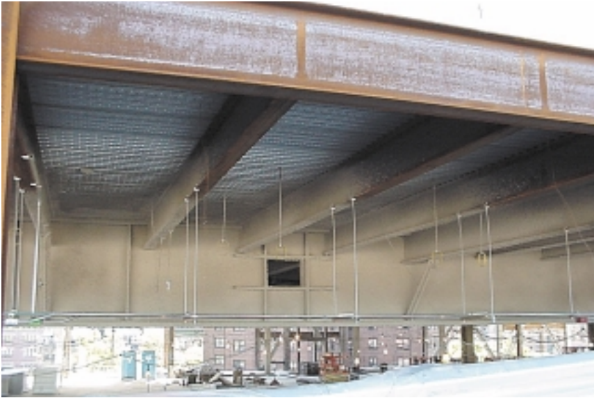
A typical built-up girder with a web penetration for mechanical systems. Spray-applied fire protection material is already in place.
