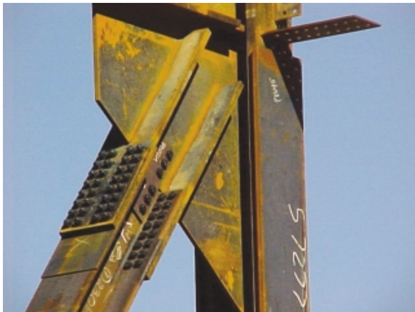
A typical connection at the top chord of a typical long-span (100') truss.
