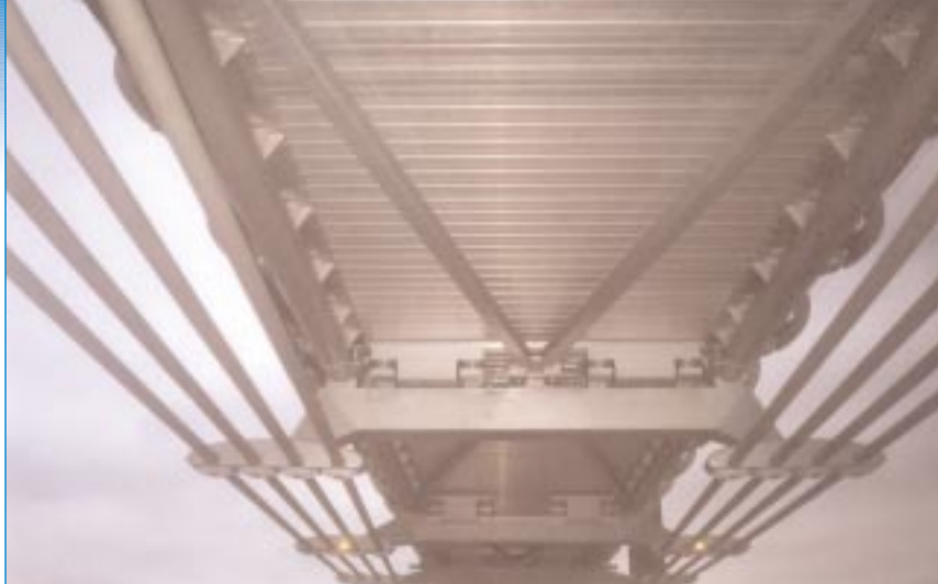
A total of 17 chevron dampers were installed. These dampers are 0.7 m (2.3') long, with a stroke of 25 mm (1").
