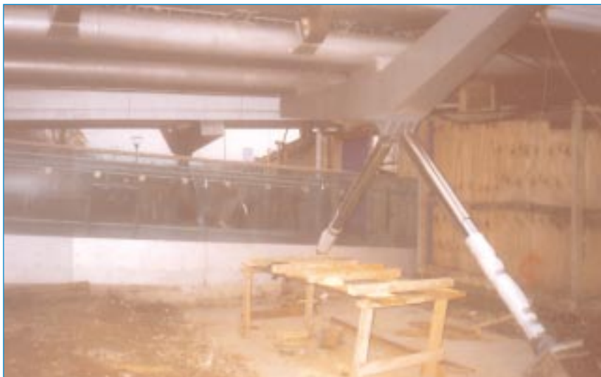
Four vertical dampers (two are shown in this photo) connect the bridge to the ground. They are 2.3 m (7.5') long, with a stroke of 275 mm (10.8").
