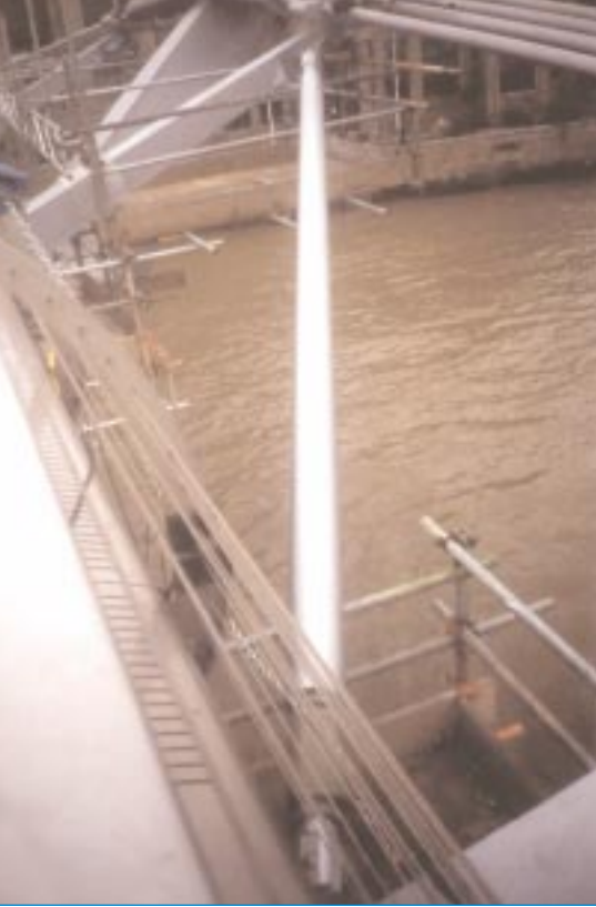
There are 16 pier dampers with a stroke of 60 mm (2.4").
