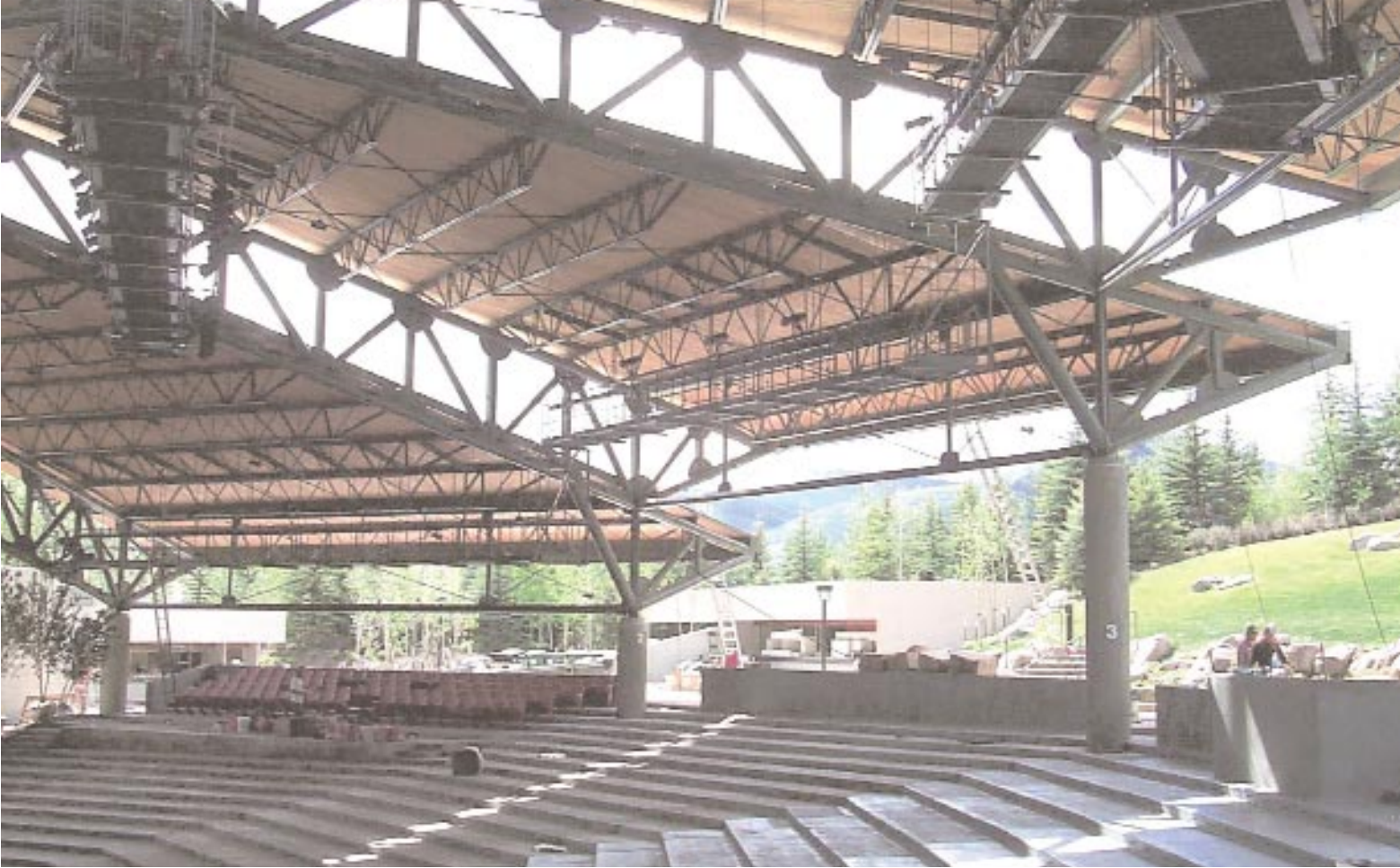
The roof structure nears completion after application of cedar plank roof deck.
