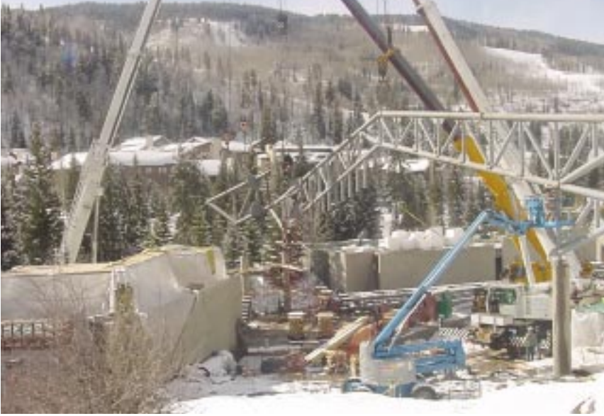
Two cranes are used to hoist the first truss into position in difficult jobsite conditions.
