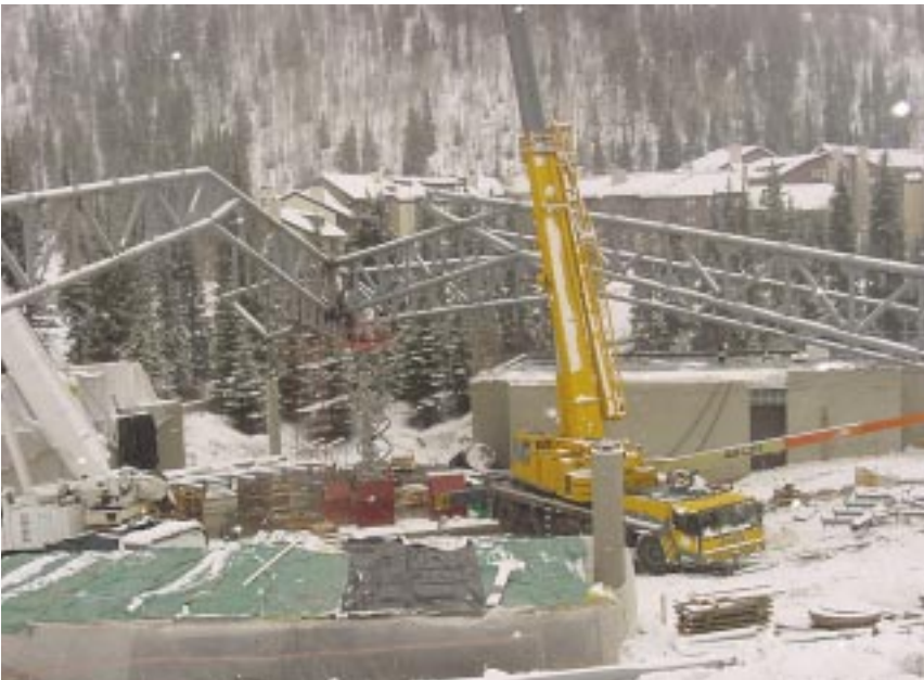
The other trusses are connected to the first truss to form the roof structure.
