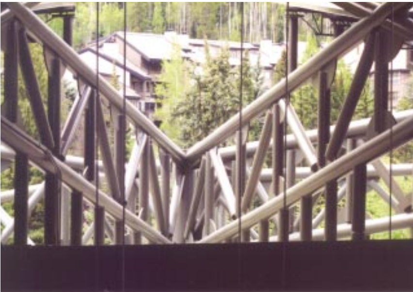
A view of the finished roof trusses as they intersect at the spindle.
