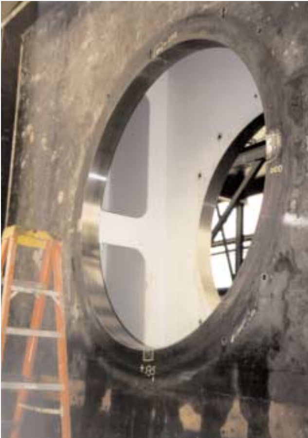
The fabricator elected to machine the completed girder for insertion of the forged trunnion hubs. The web plates are 6" thick.
