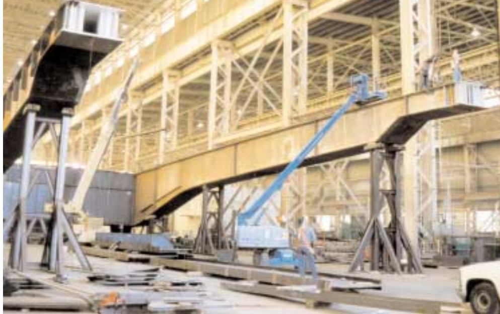
The progression of the shop assembly is key to the success of producing an assembled configuration, which can then be duplicated in the field by simply reproducing all connection configurations made in the shop.
