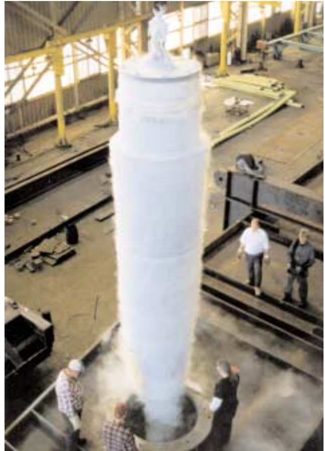
Using liquid nitrogen as a cooling medium, the 18'-5", 50-ton trunnion shafts are cooled to approximately -150° F for insertion into the main girder trunnion hubs.
