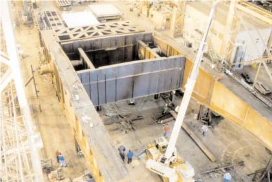
Counterbalancing in the heel section of the leaf is provided by steel ballast consisting of steel transition slabs housed in 100-ton tube box girders.
