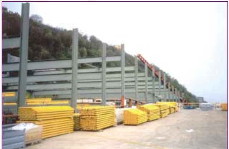
Only the upper level of the parking structure was closed during construction. This level was used as the staging area for construction materials. All the lower levels remained open for continuing parking operations with minimal interference during the construction period.
