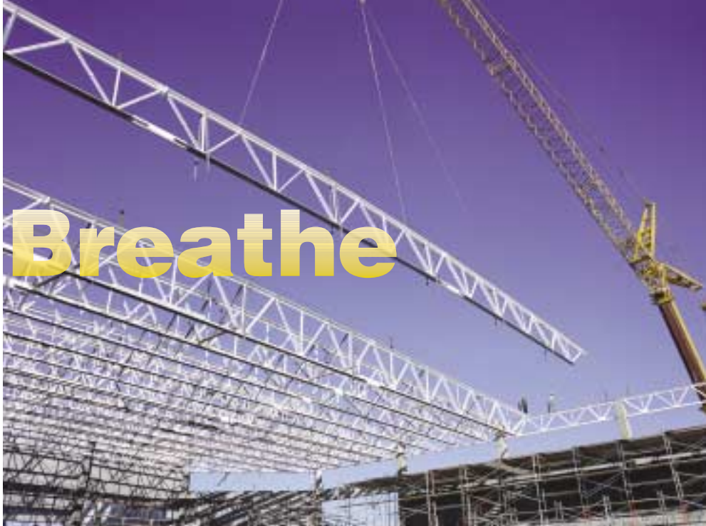
Erection of long-span joists at Angelo State University's Junell Center (San Angelo, TX).
