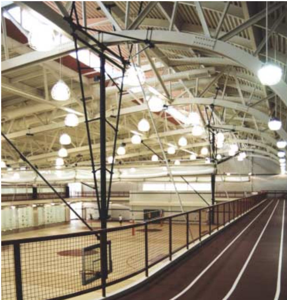
The elevated running track allows joggers and walkers to get a close-up view of the exposed steel roof framing.
