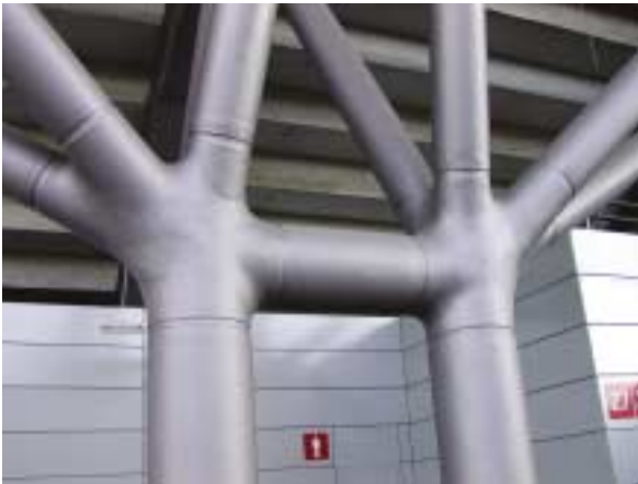
Castings are ideal for situations where several members converge, and would otherwise create a complicated and expensive fabricated connection. Column transition detail is at Stuttgart Stadium, Stuttgart, Germany
