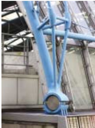
A steel casting creates a literal "hinge" connection of a three-hinged steel arch at Waterloo International Train Terminal, London, England.
