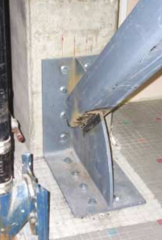
A detail at the connection between new chevron bracing and existing concrete structure.
