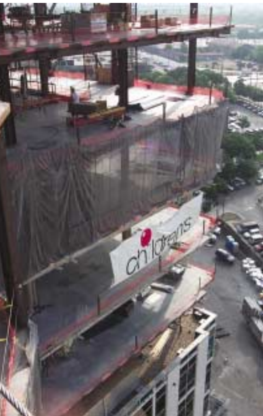
Extensive measures were taken during construction to protect existing hospital pathways from construction hazards.
