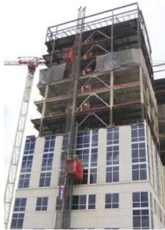
Steel tube chevron bracing was installed on both the new and existing floors to increase the building’s lateral capacity.
