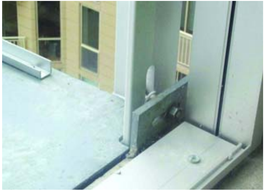
Slotted holes allow the self-supporting (for gravity) balcony structures to receive lateral support from the building while accounting for thermally induced movement.
