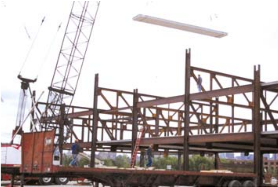
Concrete plank is placed on the staggered trusses during the construction of the Mystic Marriott.
